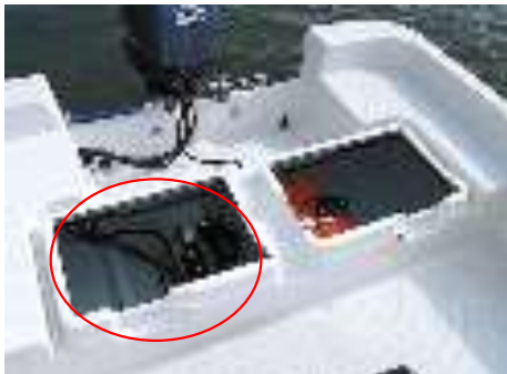
Battery space and switch
