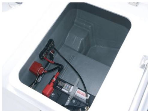
Port stern locker (battery space)
